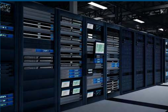
MNL1 Data Center, Philippines IFC EDGE
