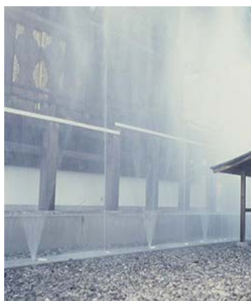
Drenchers which prevent a fire from spreading
